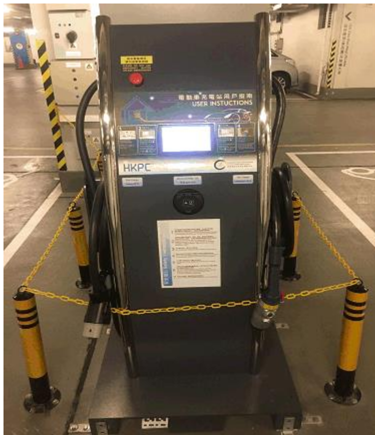
Fig. 2 – Electric Vehicle Fast Charging Station
